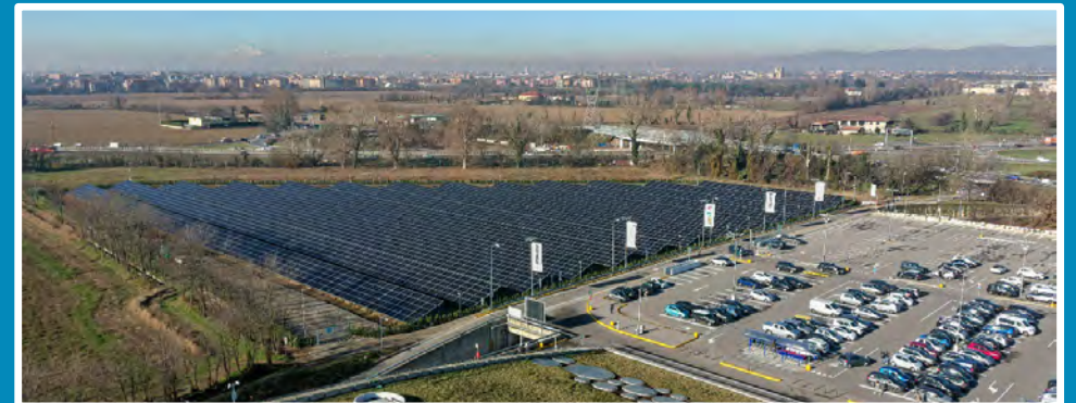
Photo: Carosello's new panels will provide around 44% of the energy needs of the common areas.
