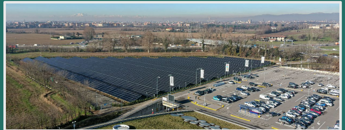
Photo: In 2024, Carosello's new panels have provided 43% of the energy needs of the common areas
